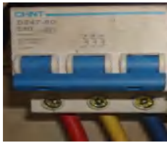
Picture 7.1 air switch
